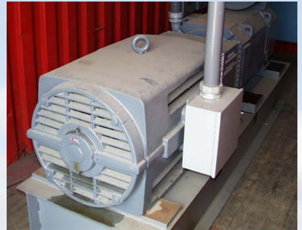
75 kW Synchronous Condenser
