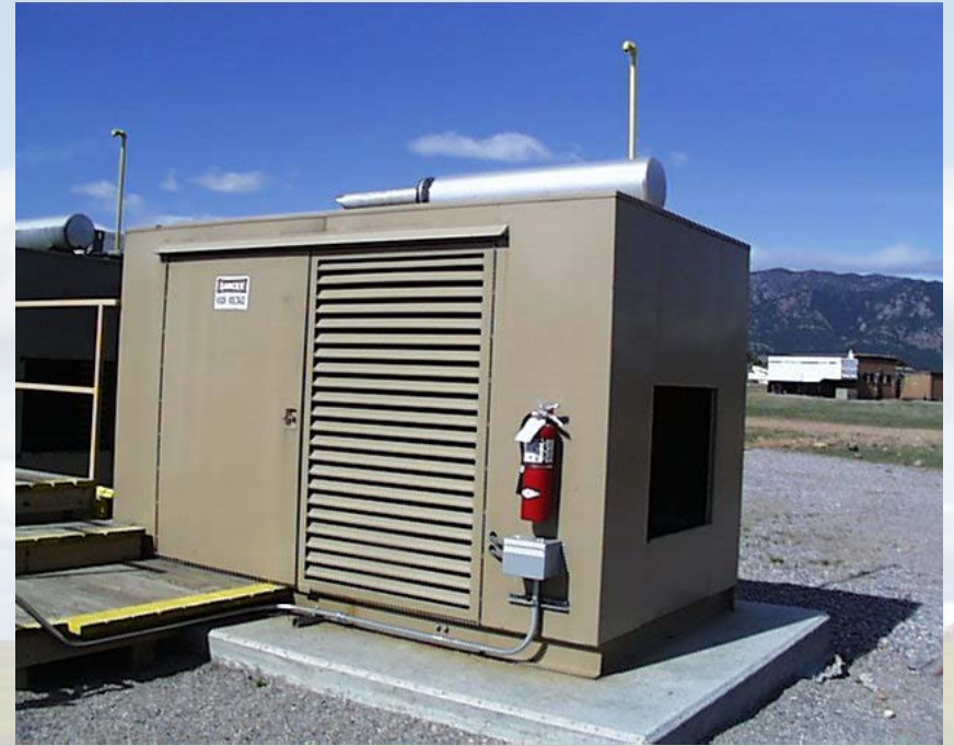
40 kW Diesel Generator
