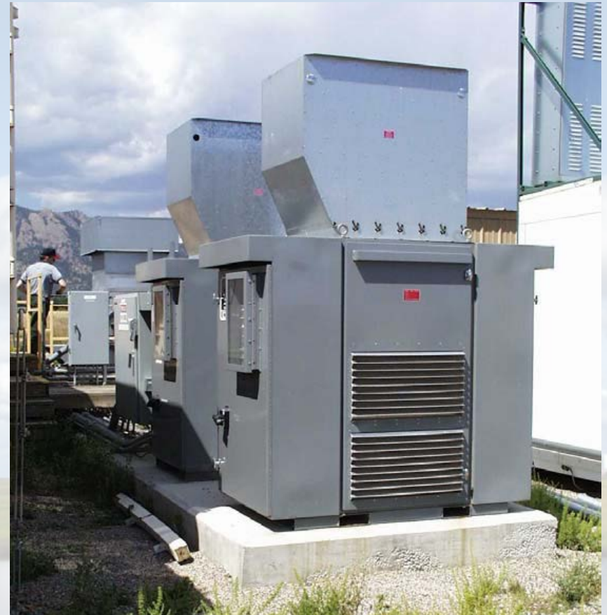
100 kW dump load
